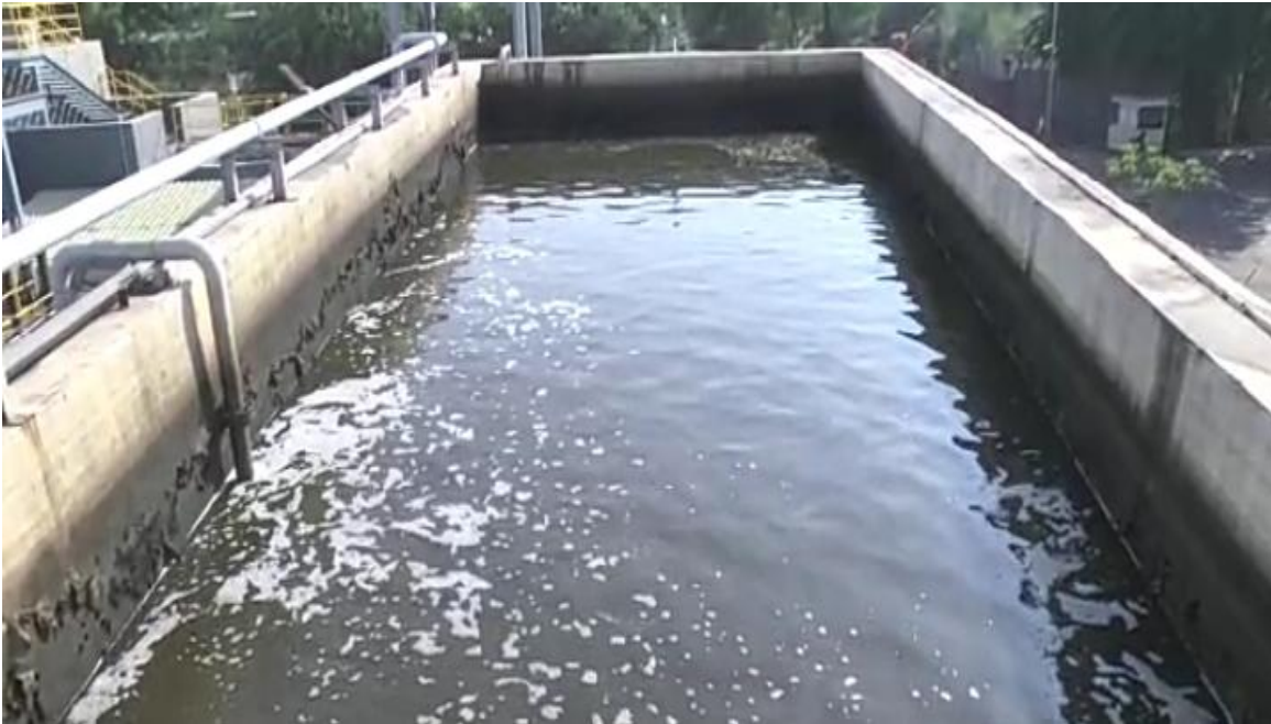
Fine Screen/Pre-aeration Tank
